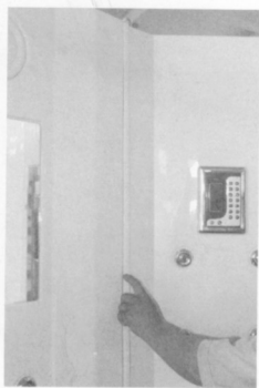
14. Put mid back board on the tray, using jointing strip fix it with back board
