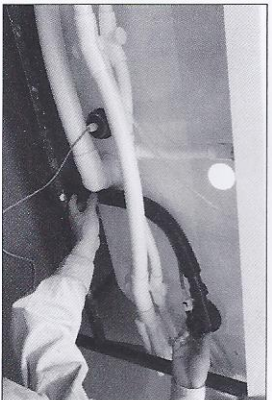
55. Let the overflow drainer near the tub.
