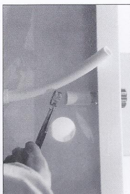
43. Seal with silica gel around inner of pipe connector from below end.
