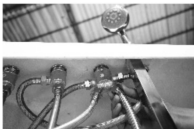
3. Distinguish water inlet pipe
