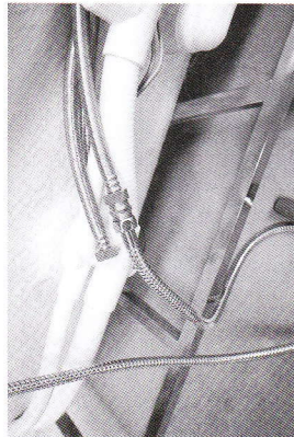
3. Distinguish water inlet pipe
