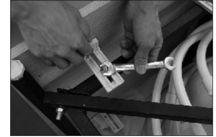
8. Use adjustable spanner to fix the "L" shape connector on the iron frame.
