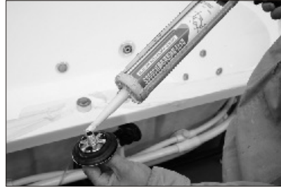
50. Seal with silica gel around the drainer as pic show and make sure no silica gel left inside of the drainer.
