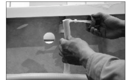
36. Seal with silica gel around inner of pipe connector from below end and outer or pipe from top end as pic shown.
